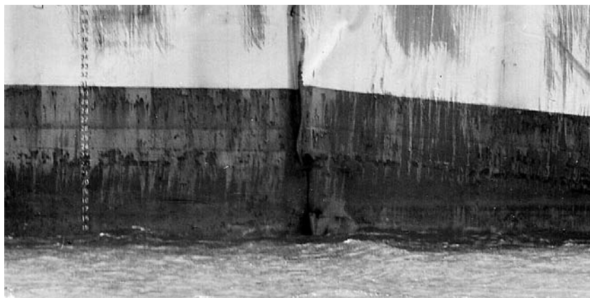
Close up of the crack in the Signa
